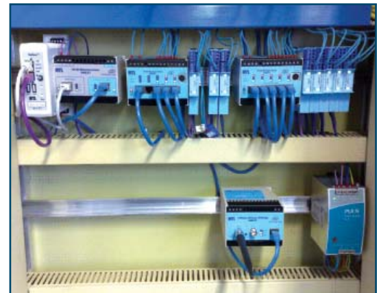
Network access hub showing Tofino™ security device, Ex i Isolator, Ex i Ethernet switch, IS power supplies and Ex i wireless interface.
